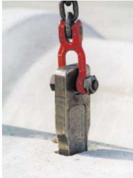
Top of pipe
